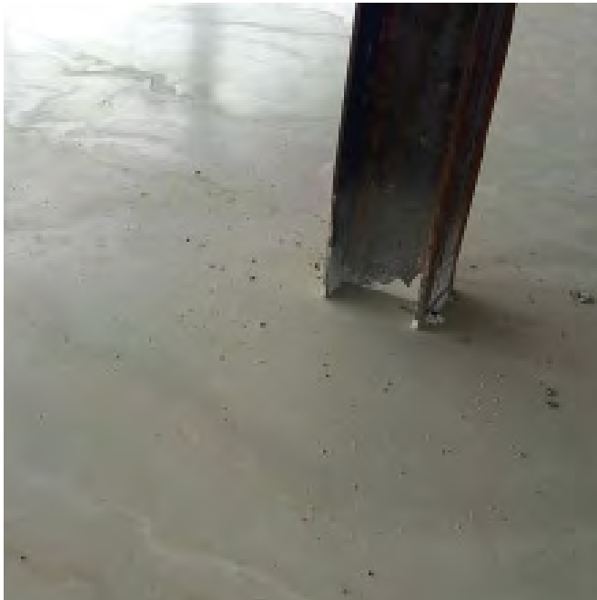
After grouting, the composite slab is complete and ready for use. The addition of any non-structural, lightweight leveling material (typically 3/4"-1") normally occurs after the building is closed and interior studs are installed.
