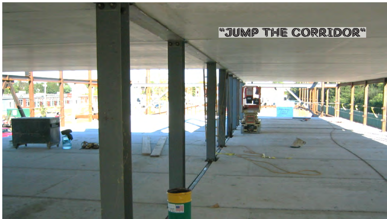
(above) D-BEAM® girders spanning the length of the building between one interior column line
